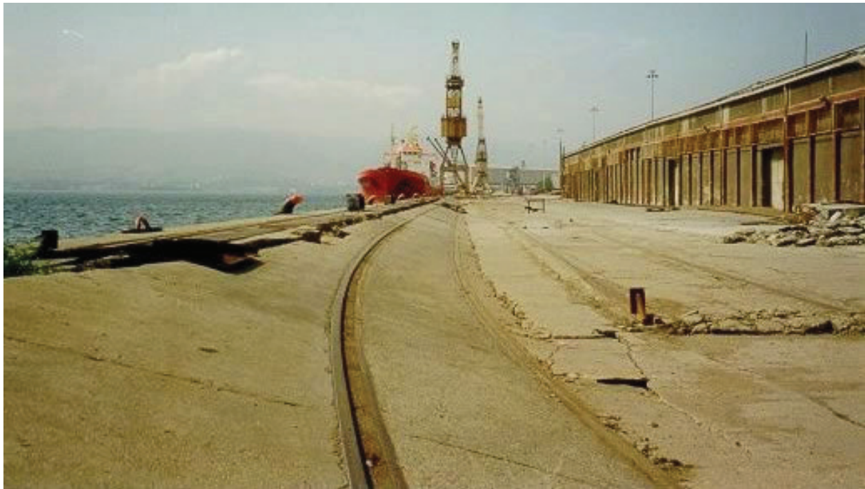
Figure 4: Damage to quay wall at Derince, Leman industrial facility. Kocaeli, Turkey Earthquake of 17/8/99. Image courtesy Earthquake Engineering Field Investigation Team (EEFIT), UK [24].
